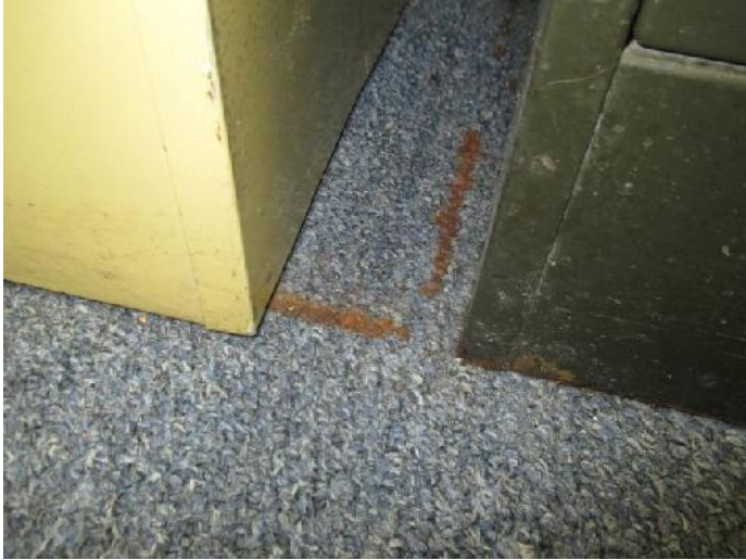
Photo #9: City Manager's Office – Water staining on carpet.
