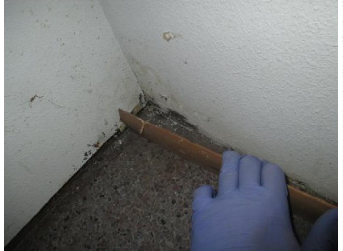
Photo #10: NE Storage – Mold growth on gypsum wallboard.
