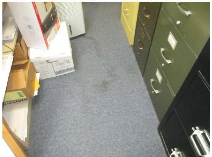
Photo #8: City Manager's Office – Water staining on carpet.
