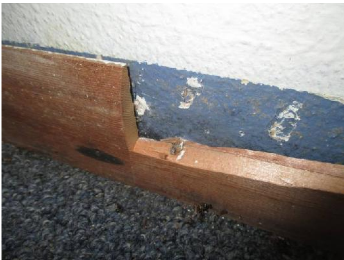
Photo #7: City Manager's Office – Mold growth on gypsum wallboard
