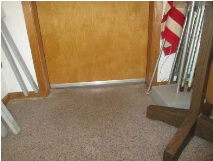
Photo #11: NE Storage – Water staining on sheet vinyl.
