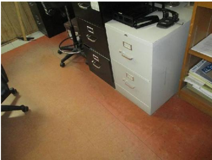
Photo #3: Building Department Office – Water staining/damage on vinyl floor tile.
