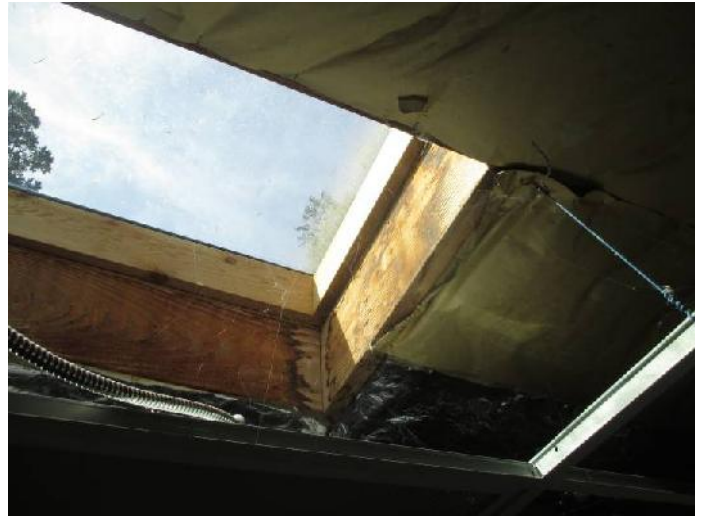
Photo #6: Building Department Office – Water staining on wood around skylight above ceiling tile.
