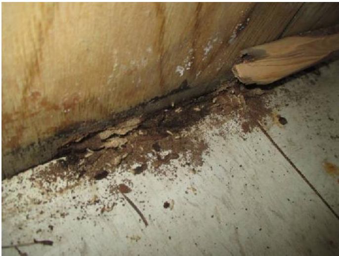
Photo #1: Building Department Office – Mold growth on wood wall paneling.
