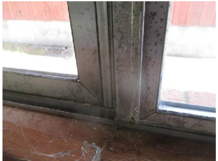
Photo #2: Building Department Office – Mold growth on window frame.
