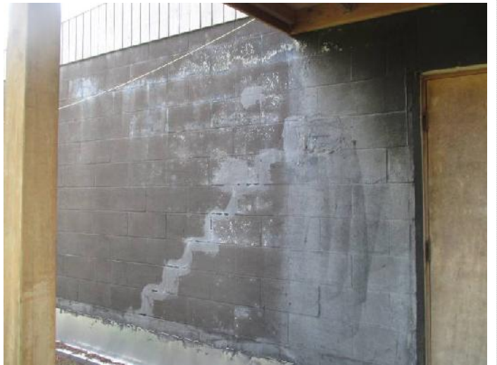
Photo #11: West Elevation – Efflorescence on CMU block.
